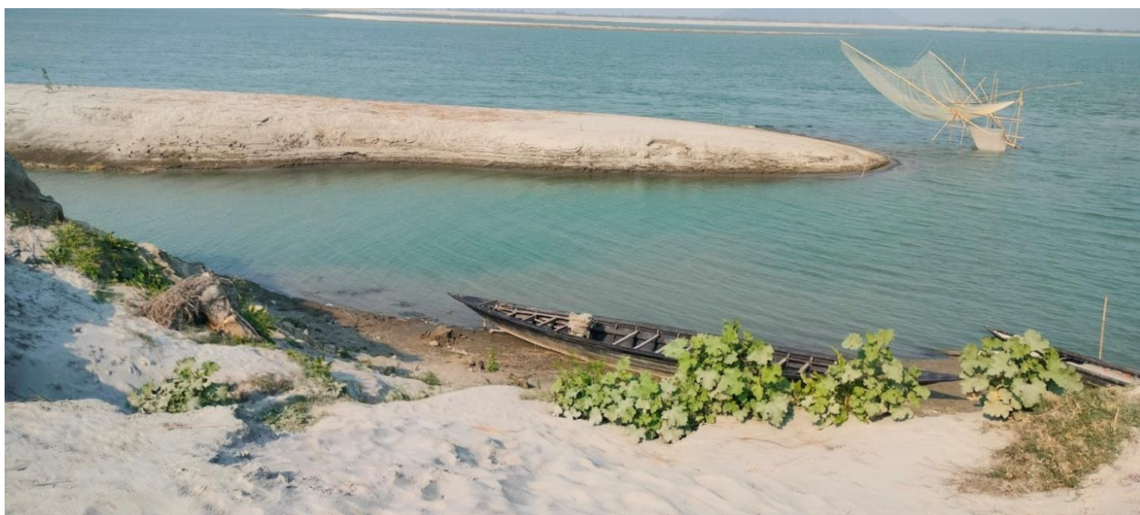
Figure 1: Embankment erosion and soil runoff at Palasbari reach
