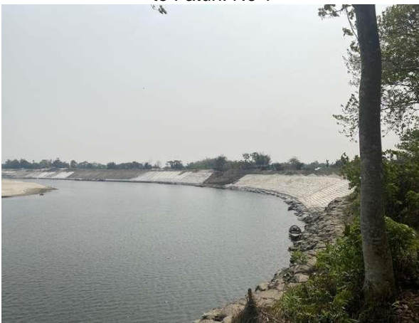
AE & FP works under progress by WRD in upstream of proposed site at Gumi
