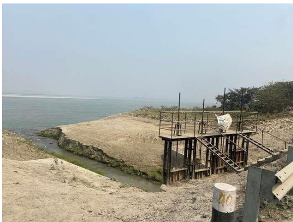
Sluice gate installed under AIFRERMIP Tranche II Kalbhog channel at Palasbari
