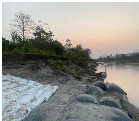
Temporary AE and FP work by WRD and at proposed site Nagarkhelia
