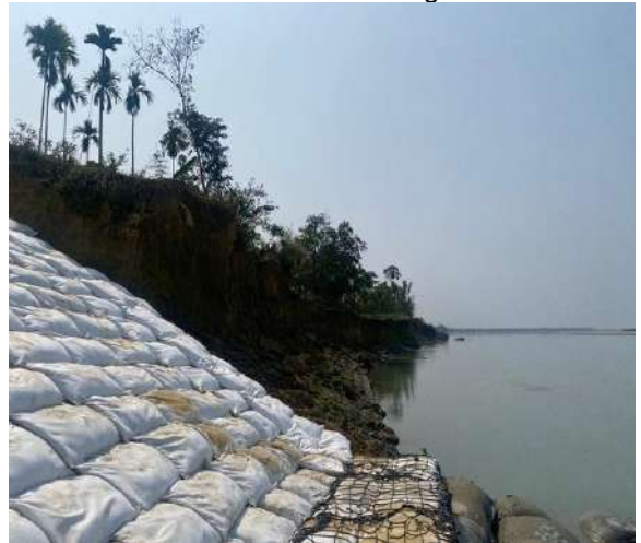
Temporary AE and FP works by WRD GoA upstream of proposed site at Baghan Notungaon
