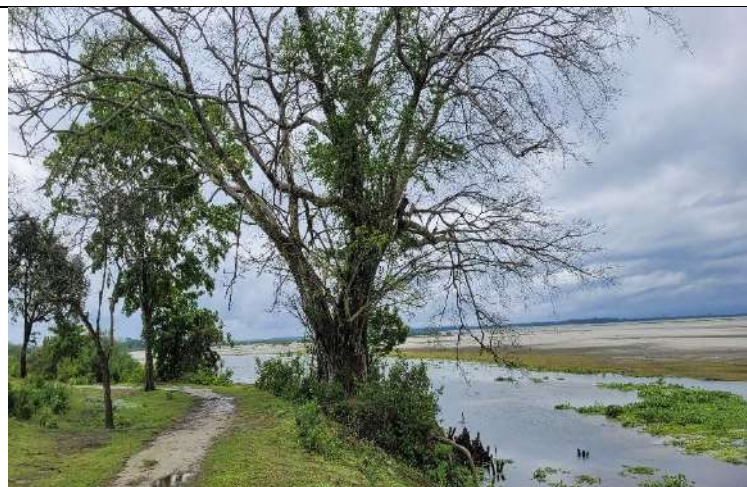
Peepal tree saved by adopting mitigation at Milanpur to Hatighuli, Tinsukia – 1500 meters bank protection work- 27.763188°; 95.564557°
