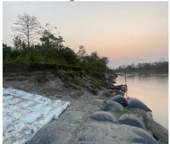
Temporary AE and FP works by WRD and at proposed site Nagarkhelia
