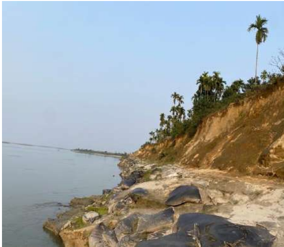
Temporary AE and FP works by WRD GoA at proposed site at Simalguri Satra
