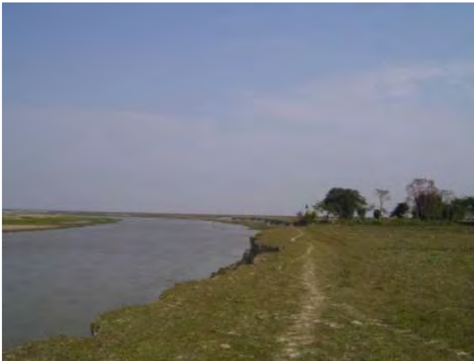
Plat 2: Erosion at Dhansirimukh
