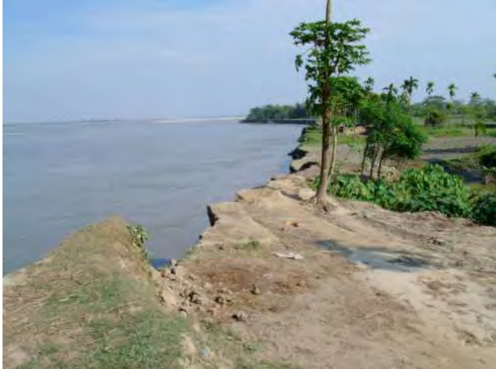
Plate 3: River Erosion near Gumi site
