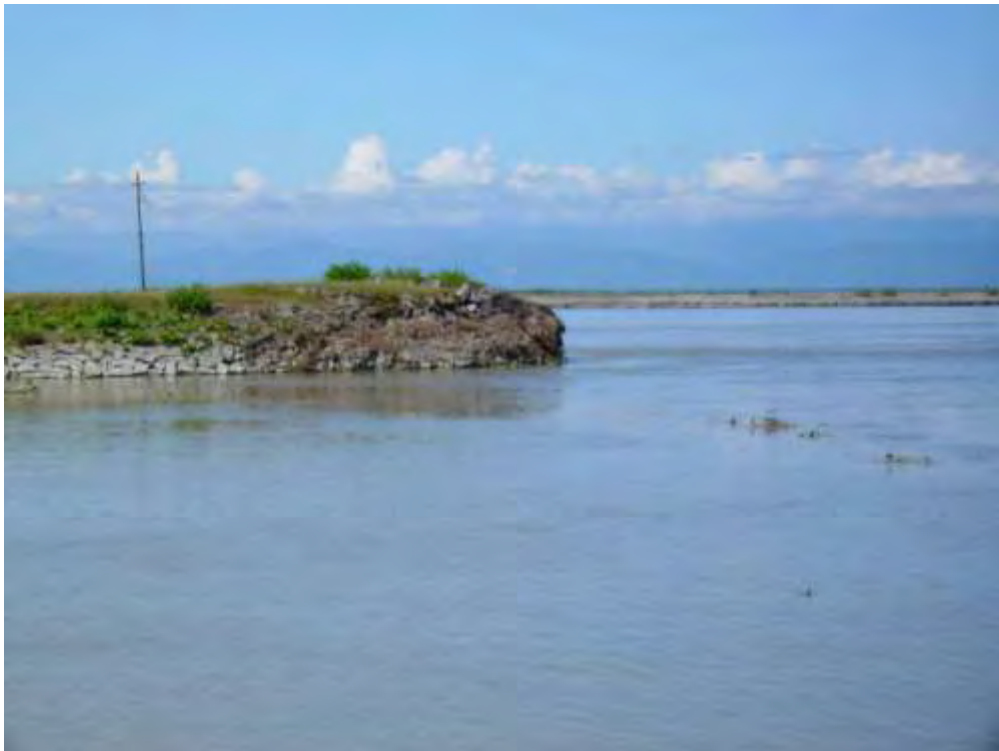
Plate 4: Existing Spur near Dibrugarh Town Protection (Damaged Spur Head)
