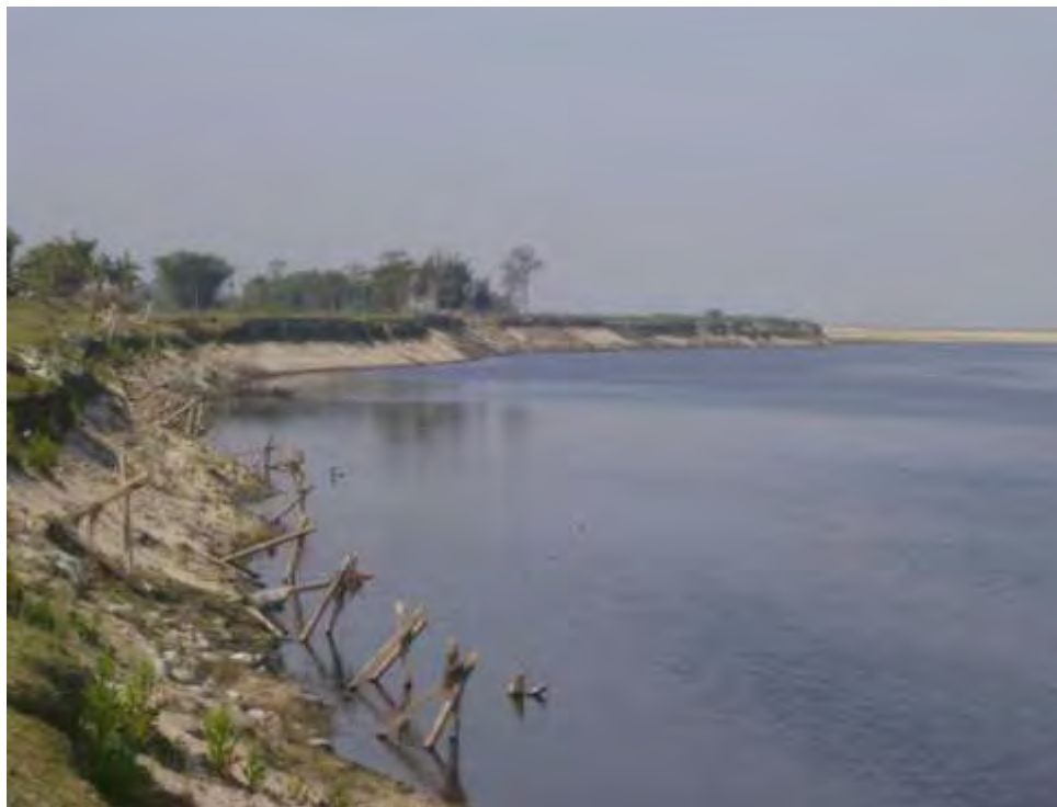
Plat 3: Erosion at Sakopara
